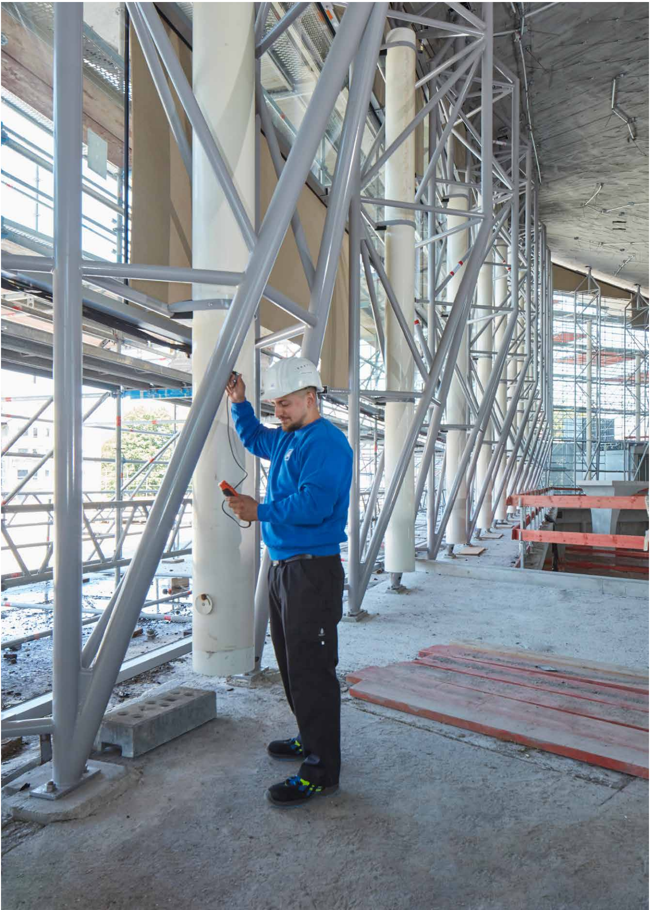
Inspection of surface protection at the indoor swimming pool Alster-Schwimmhalle in Hamburg
